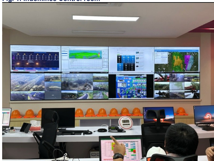
Fig. 1: Indominco Control room
