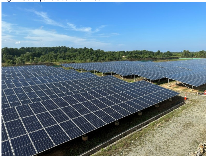
Fig. 7: Solar panels at Indominco
